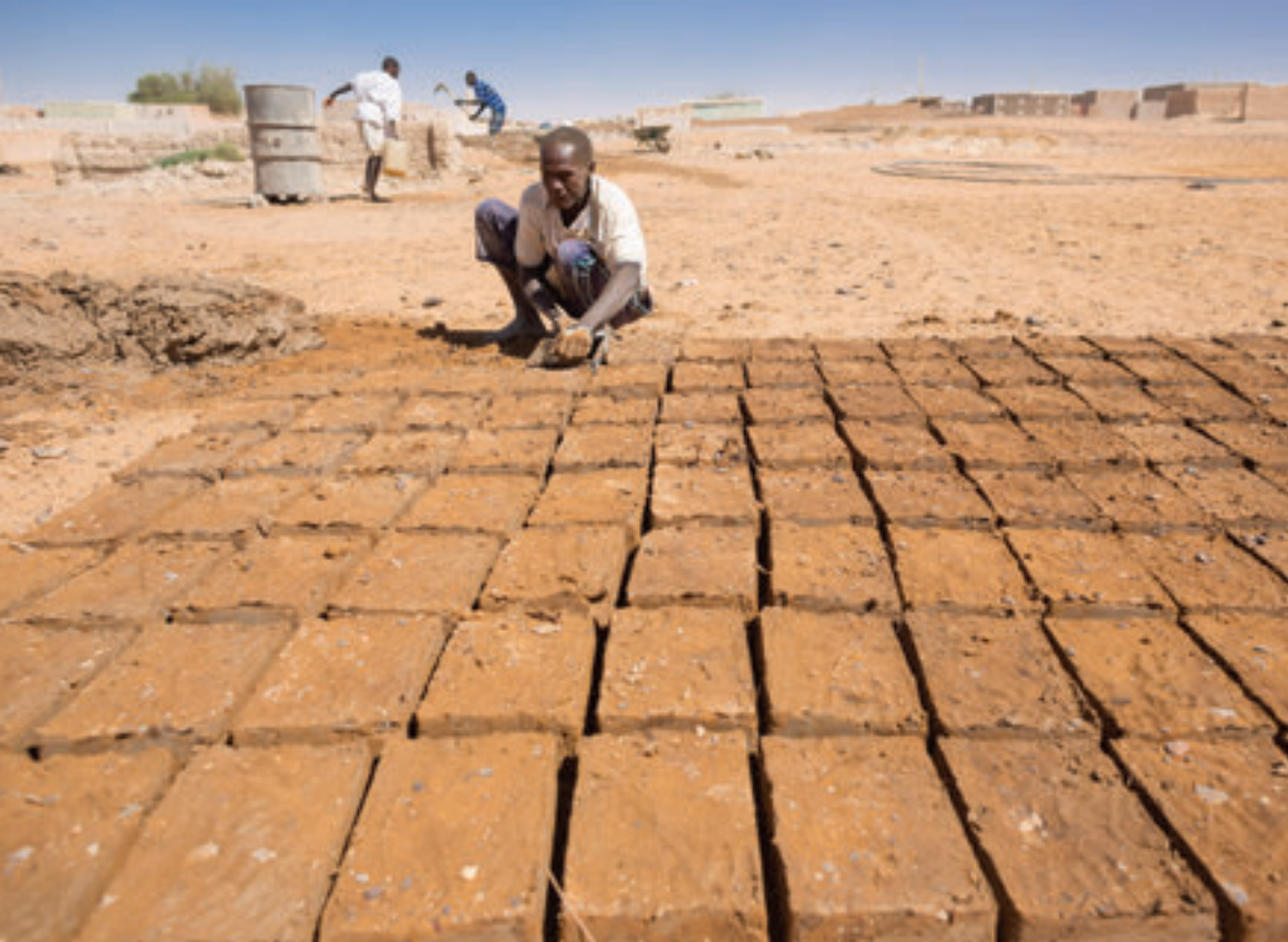
Fig. 19 Banganarti (22.11.2017), the beginnings of building a new house. The crushed material from the demolished old building is poured over with water, and the muddy substance formed in this way is used to produce unfired bricks for a new one. Photo by Andrzej Chojnacki
