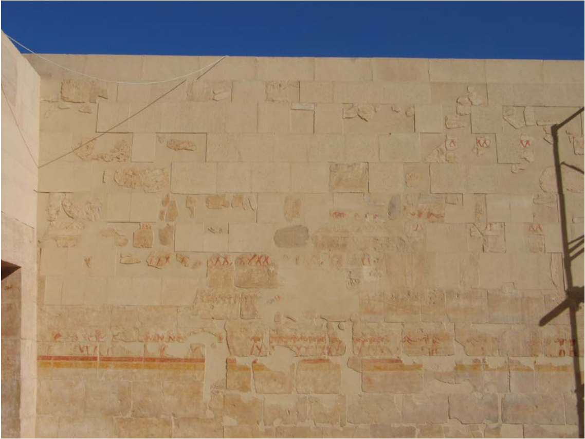
Fig. 1. Remains of the original shape of the north wing of the east wall of the Upper Courtyard in the form of vertical joints through five layers of blocks (Phot. J. Iwaszczuk).
