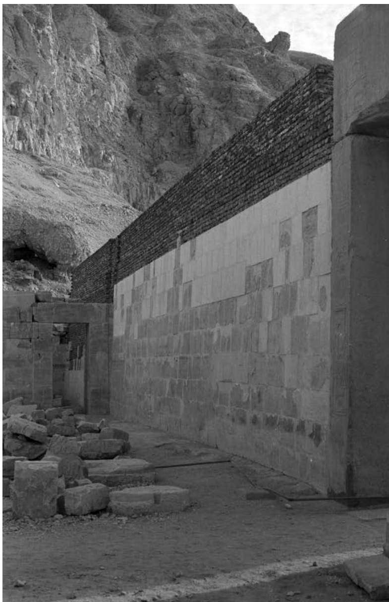
Fig. 32. Final effect of the reconstruction work in season 1976/1977 (PCMA UW | inv. no. DBAH.1976-1977.006.239).
